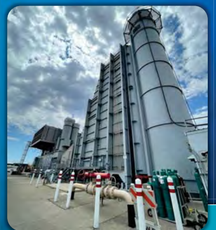
Industrial Combustion Boilers/Process Heaters/ Refineries/EGUs/Etc.
