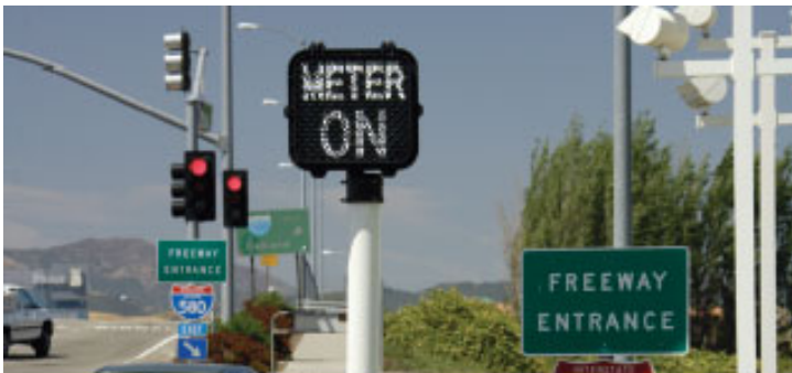
Caltrans programmed freeway onramp traffic lights to alternate so cars merge once onto the freeway, eliminating the additional merge within the onramp.
