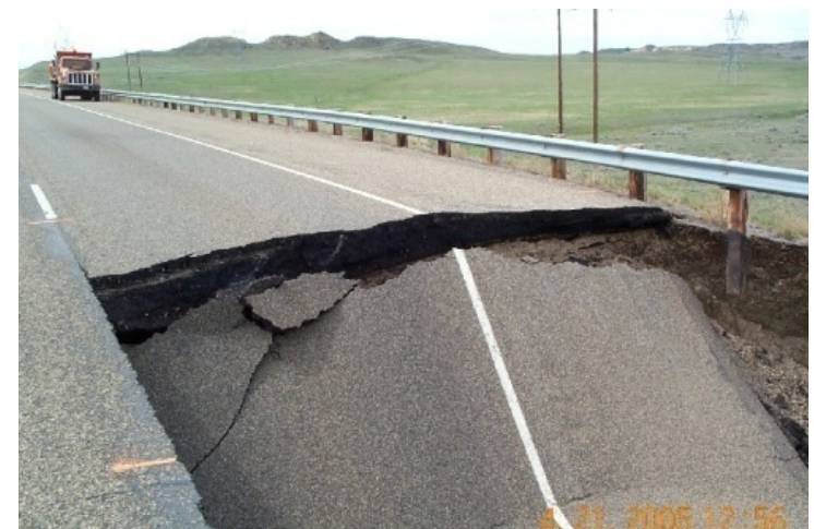
Failed culvert street view
