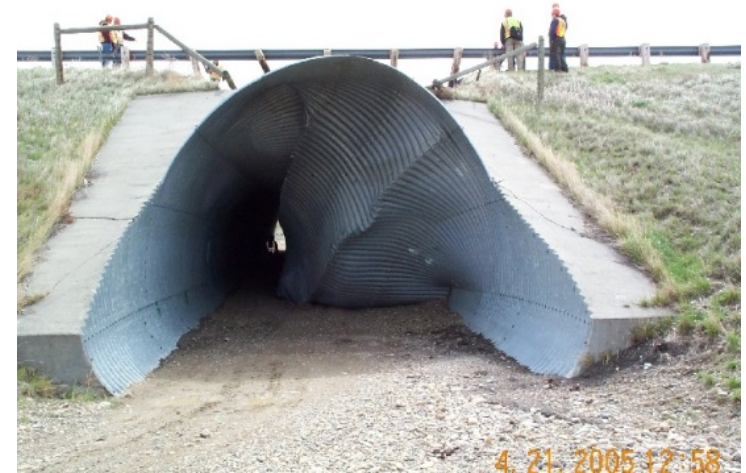
Failed culvert entrance view
